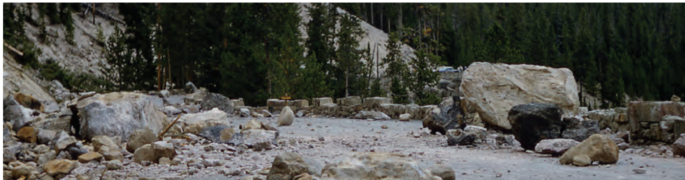
Approximately 1,000 to 3,000 earthquakes occur each year in the Yellowstone area; most are not felt. The 1959 Hebgen Lake earthquake (M7.3) caused significant damage to park roads, shown here near Gibbon Falls.
