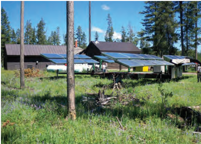
This portable photovoltaic system at Bechler provides power during the summer season, meeting 90% of the site’s electrical needs.
