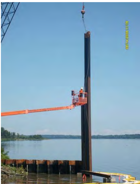
A portion of the Willis-Semet barrier wall is installed along the lakeshore.
