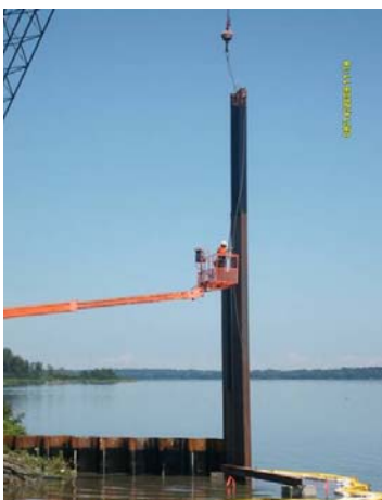
A portion of the Willis-Semet barrier wall is installed along the lakeshore.
