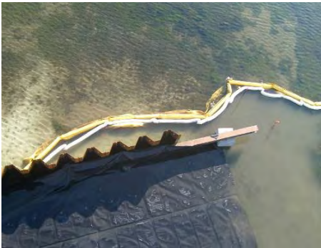
A silt curtain reduces turbidity in the water, as shown in the above photo taken during the installation of the Willis IRM Barrier Wall. A curtain extends to the bottom of the lake to contain any resuspended material.
