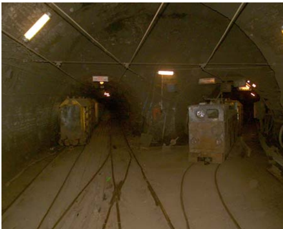
Plate 10.2 A shaft section of the main pit in Lyukóbánya secured by a concrete frame and steel rings (Sütő 2003)
