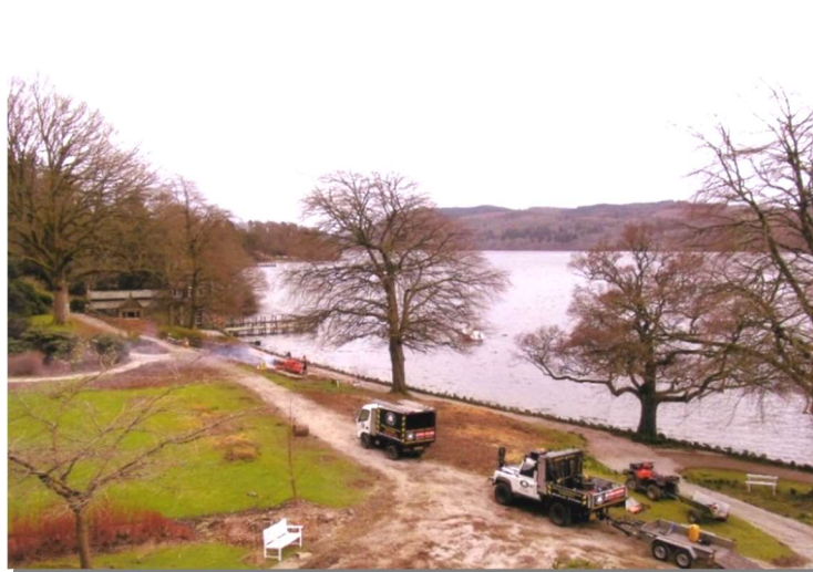
Figure 11.I.10 In the spring of 2018, clearance work was undertaken in the garden by Will Hicks, Tree Surgeons, which returned the house to having a much more open aspect, the only remaining original plantings being the two mature Fagus sylvatica 'Purpurea' — copper beech and a smaller Quercus robur — pedunculate oak.
