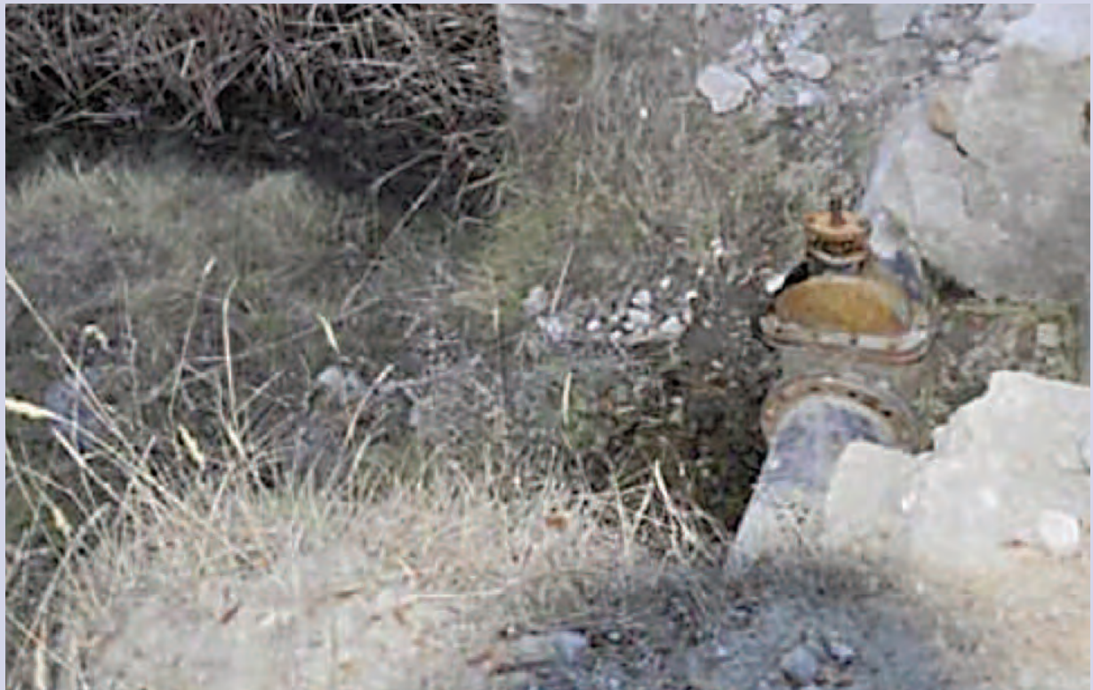
Exhibit 3.40: Valves from the Water-storage Tanks
