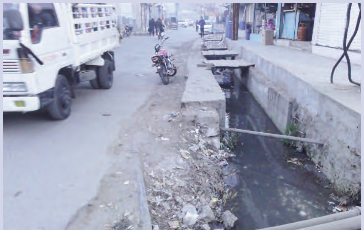
More open drains in the city center.
