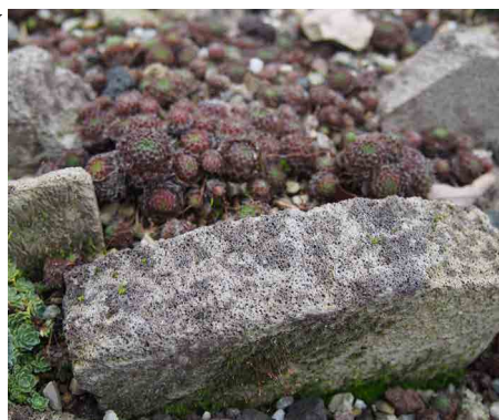
Weathered aircrete blocks after a couple of years in the garden.
