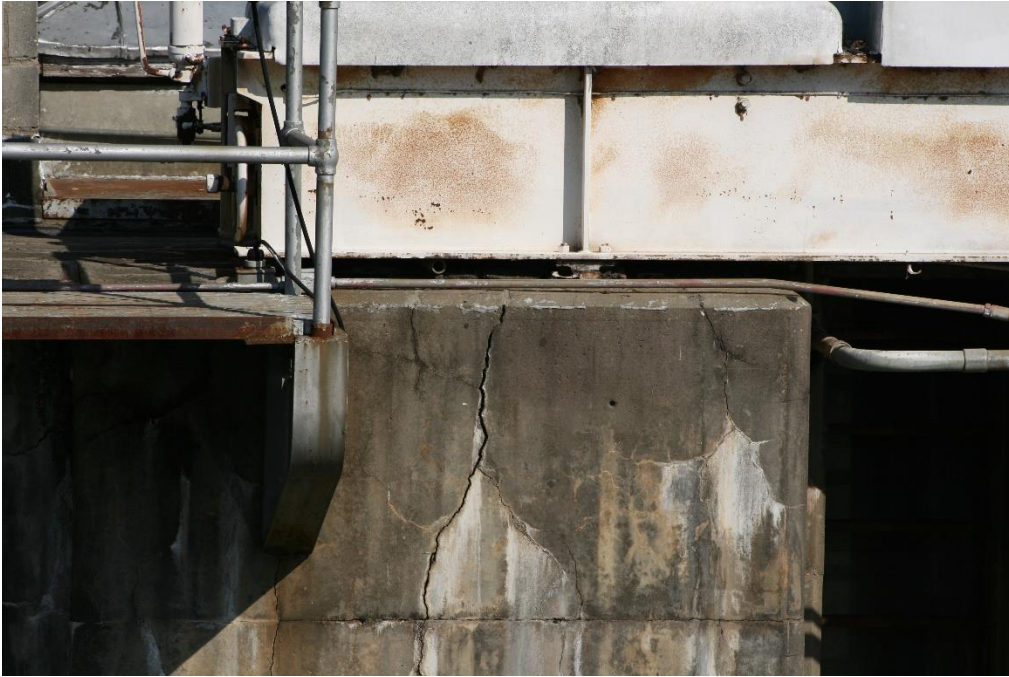
Figure 4: Cracks in NSBLD
