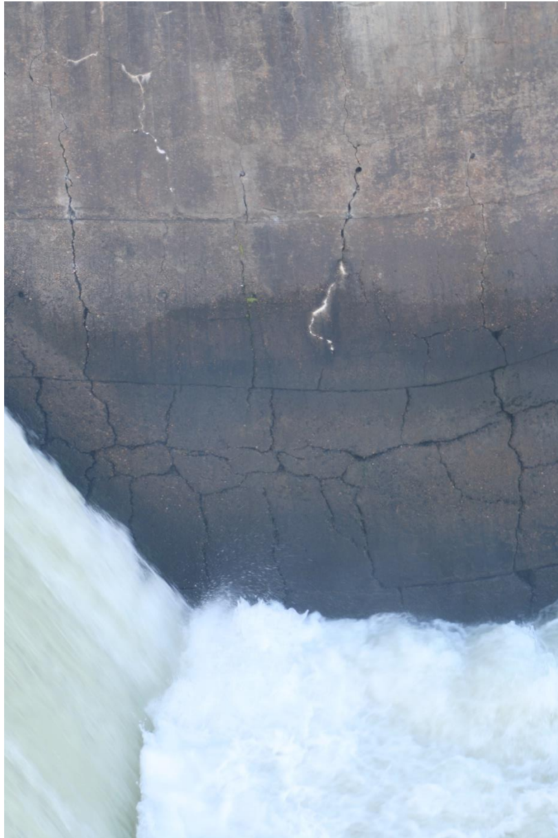
Figure 5: Cracks in NSBLD
